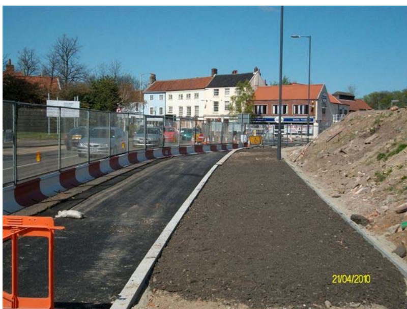
Pitt Street, looking north showing the carriageway widening and the new footway/cycleway
